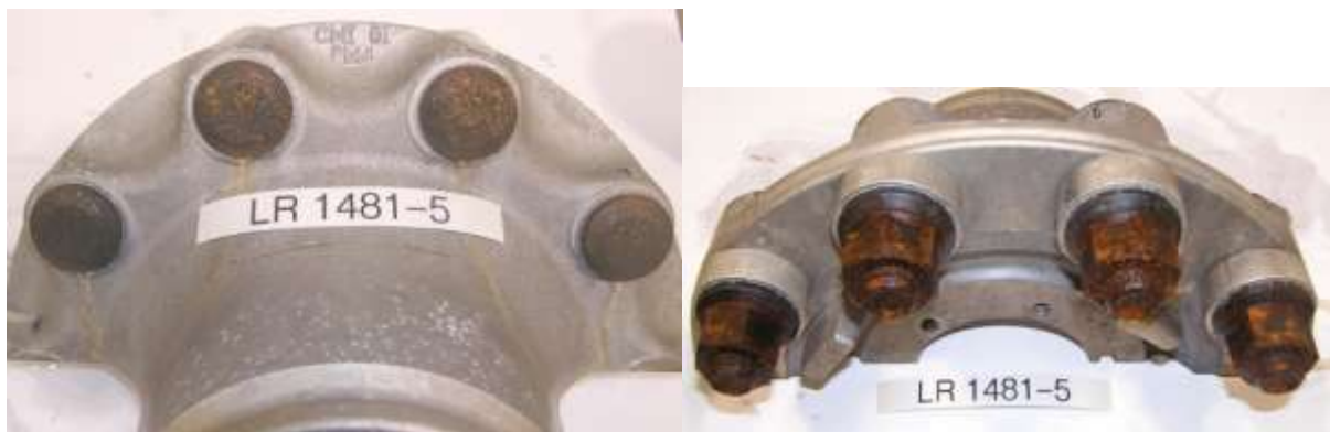
40 Cycles – Group 5 – Current Aluminum Wheel Manufacturer Technology Threads totally involved in red rust. Extensive base metal (red rust) corrosion in damage areas on nuts.
